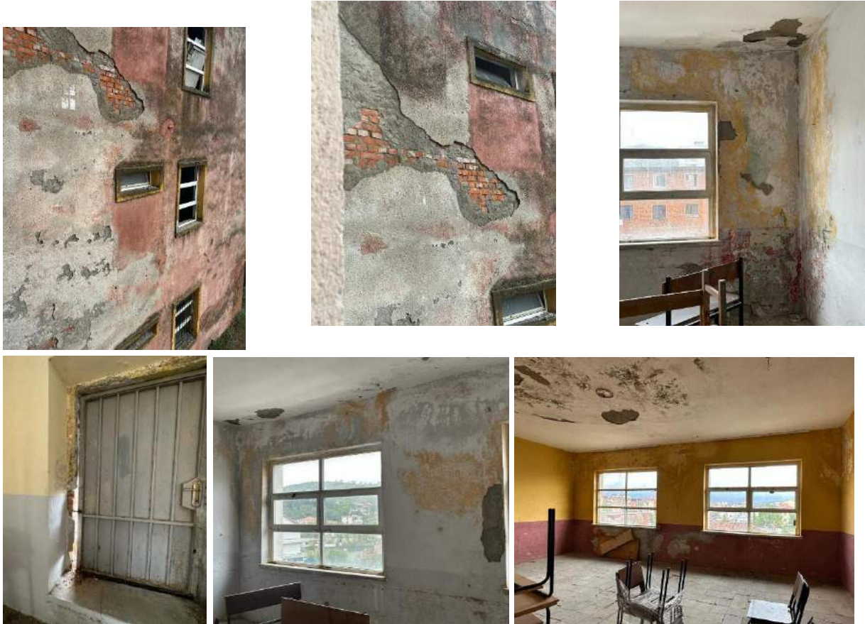
Figure 3 Pictures depicting the current state and deterioration
